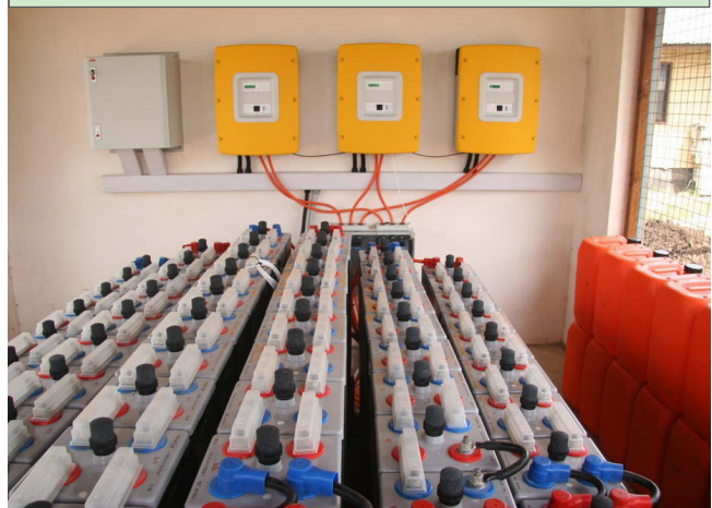
Figure 53: Flooded deep discharge lead-acid battery bank feeding three SMA Sunny Island inverter/chargers. Image Source: © DreamPower Solar.
