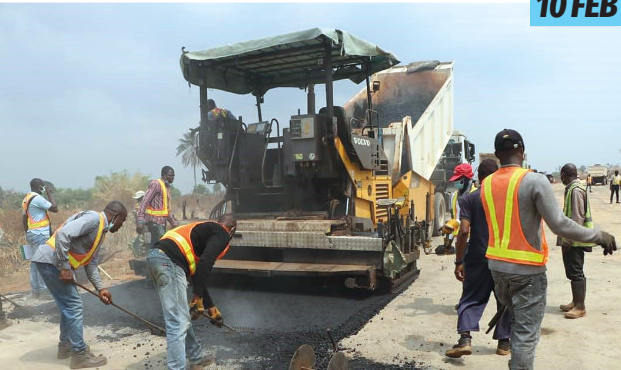
Personnel of RCC Niger Limited at work on the dualisation of Lokoja-Benin Road, Obajana Junction-Benin City, Section IV, Ehor-Benin City in Edo State, Contract No. 6138 (Sukur Project)
