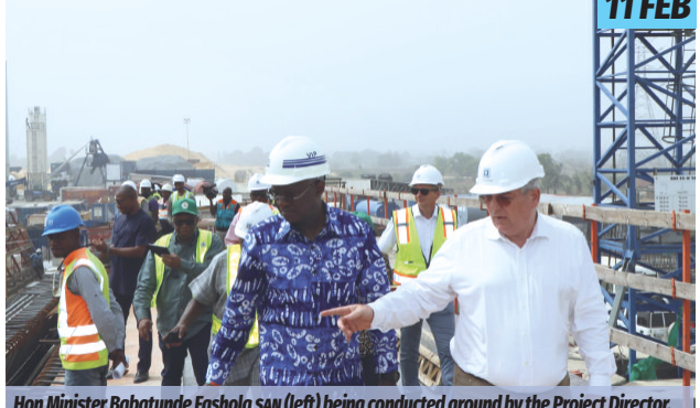
Hon Minister Babatunde Fashola SAN (left) being conducted around by the Project Director, Engr. Friedrich Josef Wieder (right) during the inspection of the 2nd Niger bridge in Anambra and Delta State
