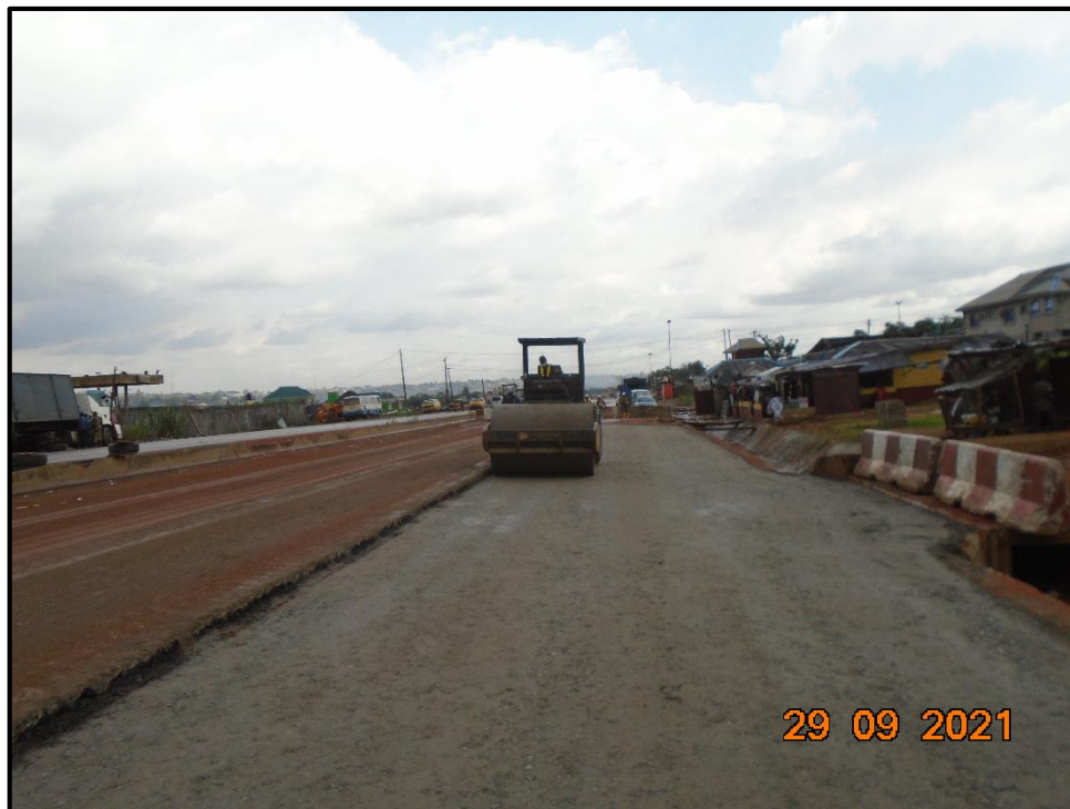
SPREADING AND COMPACTION OF STONE BASE IN PROGRESS BETWEEN CH 26+000 AND CH 26+070 (LAGOS BOUND)
