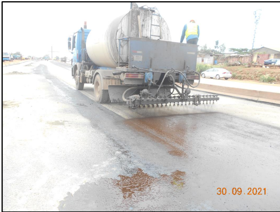
SPRAYING OF MC1 AS PRIME COAT ON CARRIAGE-WAY BETWEEN CH 21+924 – CH 21+940 AND CH 21+270 – CH 21+965 (LAGOS BOUND)
