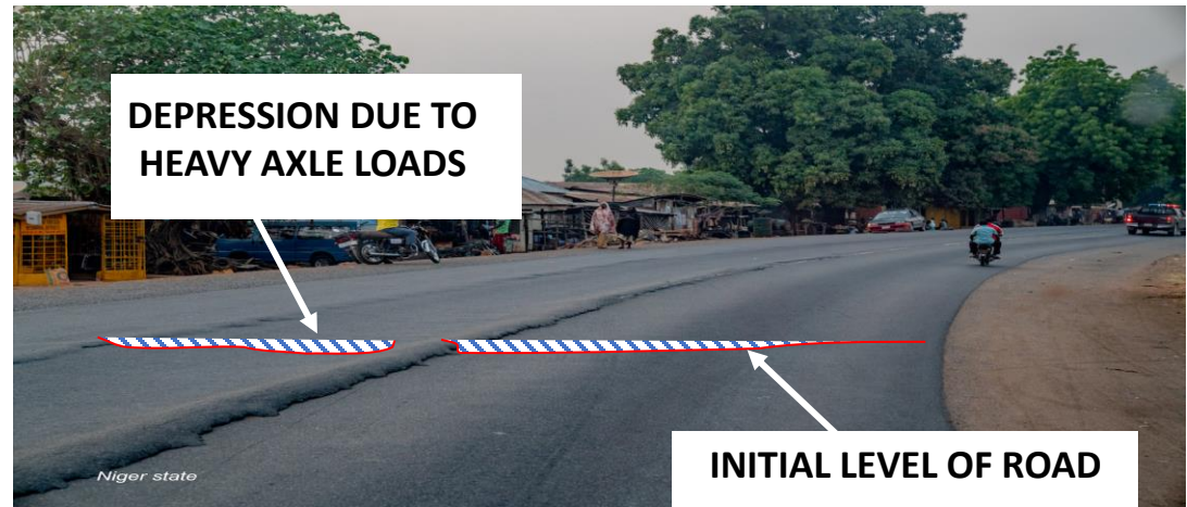
RUTTING DUE TO HEAVY AXLE LOAD
