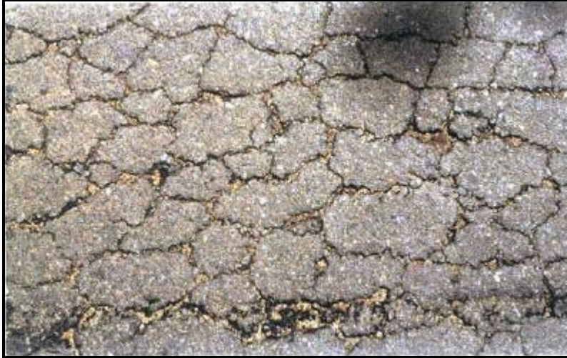
Figure 23: Alligator / Crocodile Cracking
