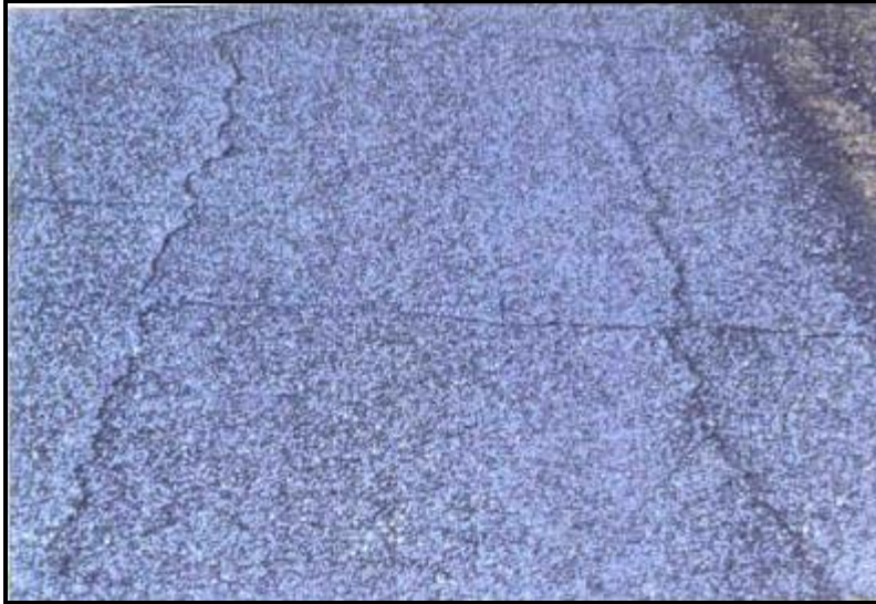
Figure 24: Shrinkage or Stabilisation Cracks
