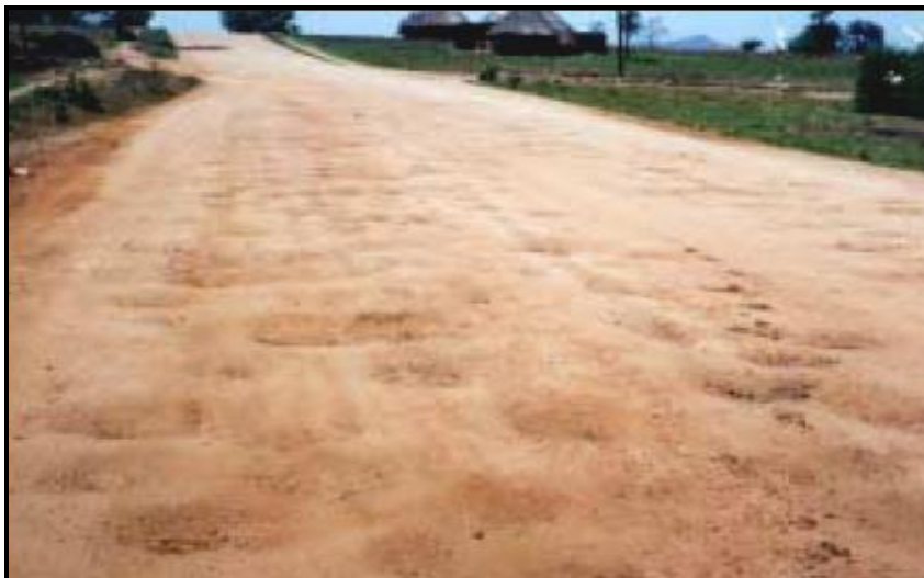
Figure 27: Potholing of Gravel Roads
