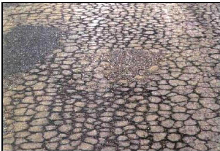
Figure 25: Severe Surface Cracking
