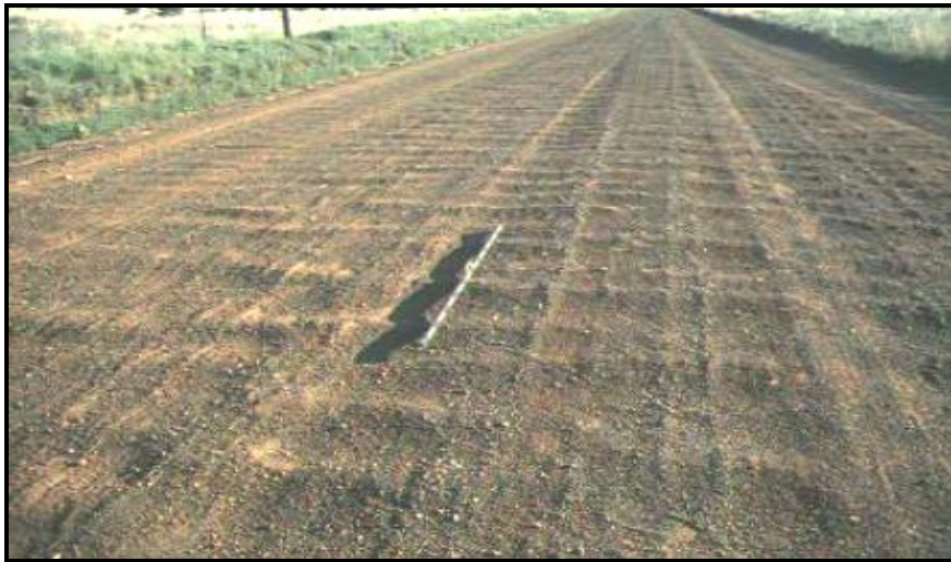
Figure 29: Corrugation of Gravel Surface
